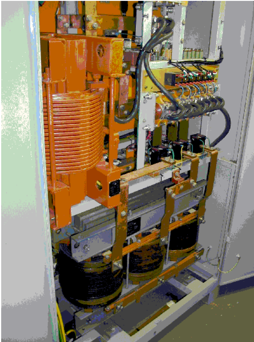
Figure 9.7 : A 500A/100V power supply made by Yerphi which is working at DESY (HERA ring). The transformer, choke, thyristors and the water cooling pipes are shown in the picture.
