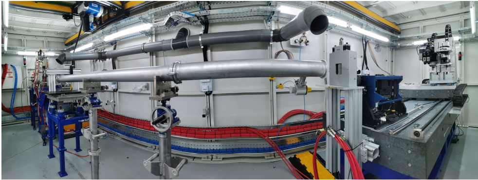
Fig 1.4: The BEATS beamline was inaugurated on 6 June 2023. It will receive its first users in 2023. Its full-field X-ray radiography and tomography capabilities extend the scientific possibilities of the Facility and the research opportunities in the region.
