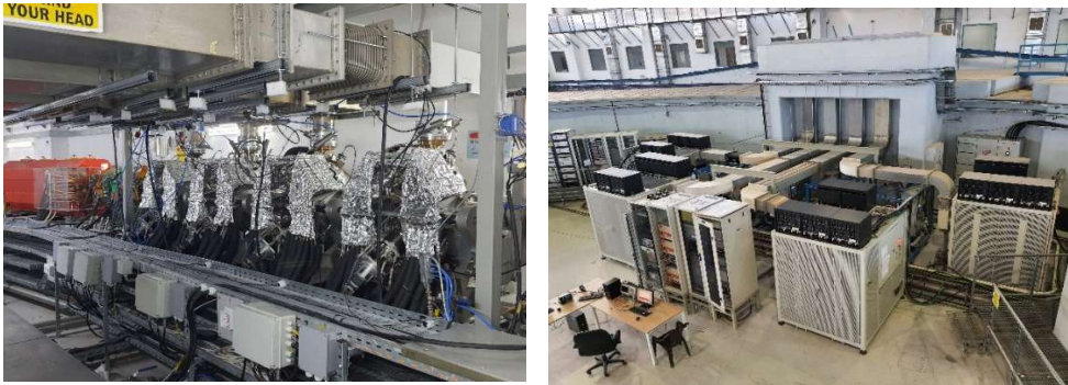
Fig 1.6: RF cavities (left) and RF solid state amplifiers (right).
